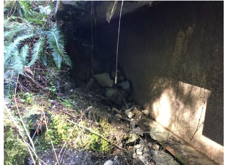
Upstream left bearing buried with sediment
