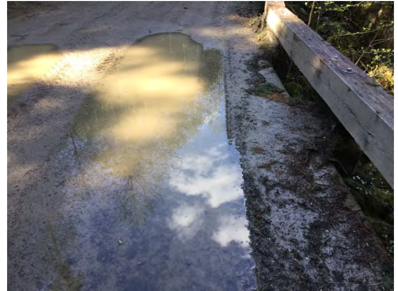
Water pooling deck due to sediment accumulations
